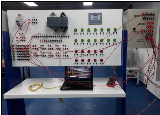
Fig. 1. Tablero de control PLC
